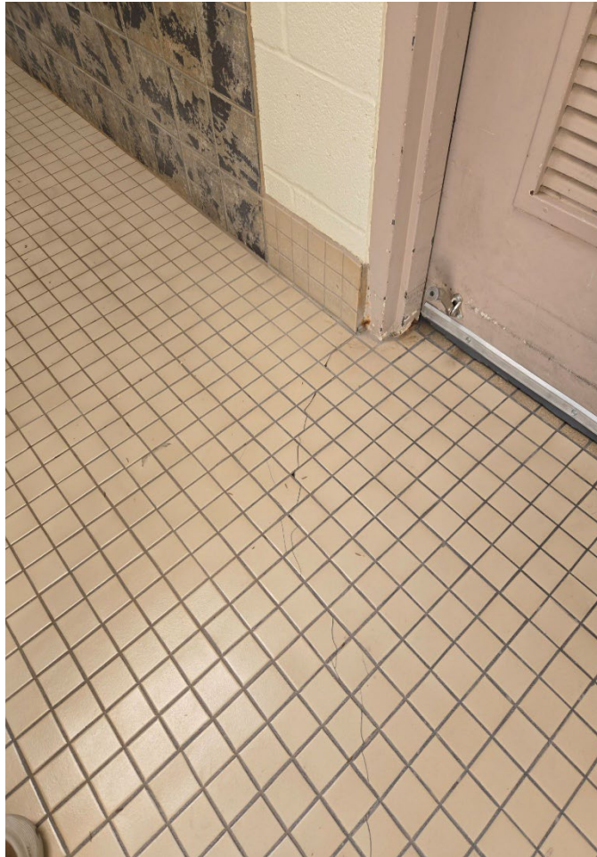
Photograph 3: Bath House - Floor Tile Crack
