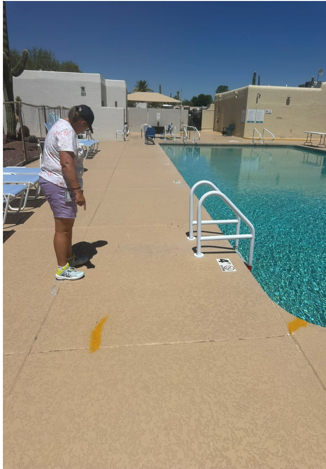
Photograph 9: Concrete Desc - Slab Settlement and Joint Separation
