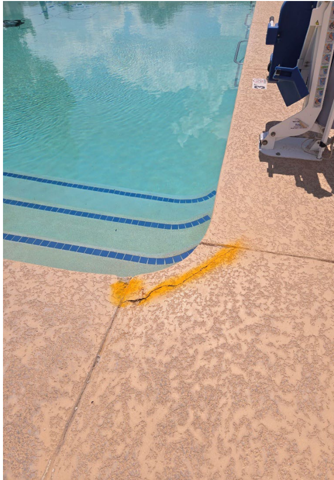
Photograph 7: Concrete Deck - Corner Crack
