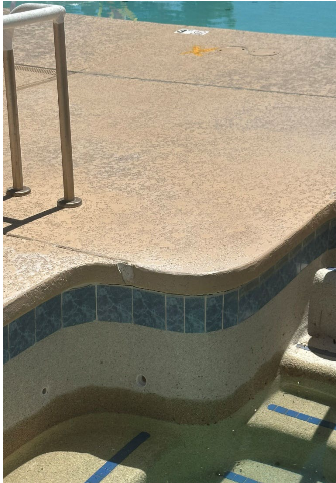
Photograph 11: Spa - Deck Separation
