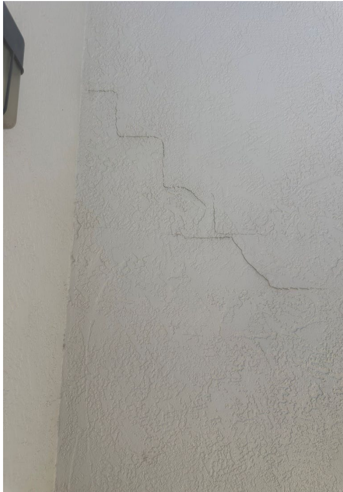
Photograph 5: Bath House - Stepping Crack in Exterior Wall
