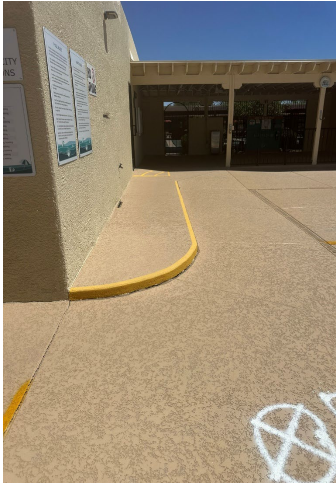
Photograph 8: Concrete Deck - Slab Settlement
