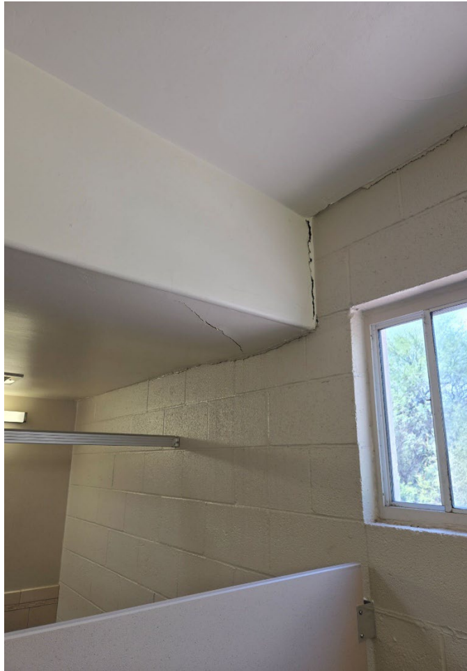
Photograph 1: Bath House - Ceiling and Wall Separation
