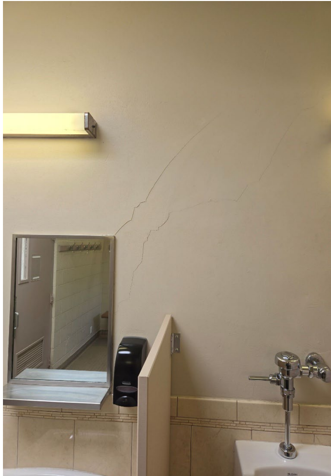
Photograph 2: Bath House - Diagonal Crack in Dry Wall
