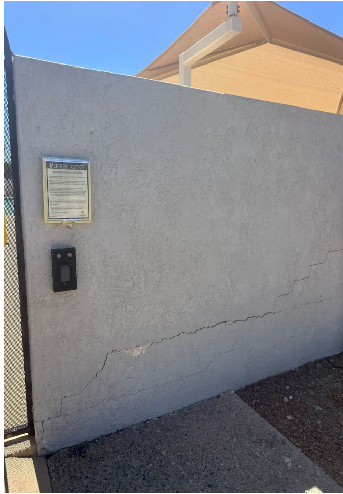
Photograph 12: Equipment Area - Horizontal Crack in Masonry Wall
